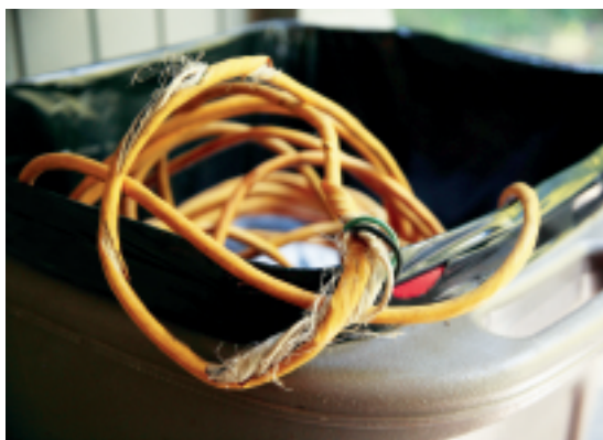
Dispose of frayed, cracked or damaged cords and replace them immediately.
